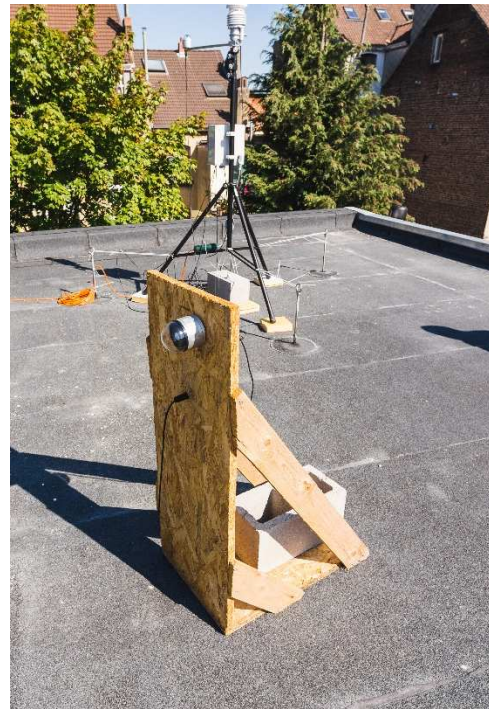
Figure 36 : Solar radiation sensor on the roof
