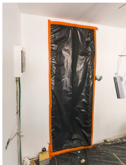
Figure 30 : Sealed bathroom door
