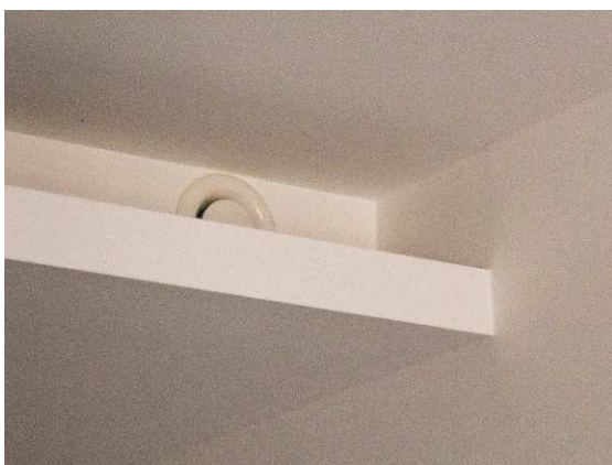
Figure 25 : Ventilation outlet unobstructed during experiment
