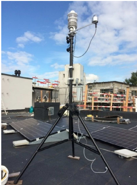
Figure 34 : Weather station on the roof
