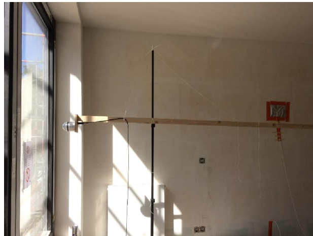
Figure 26 : Pyranometer in unit BU
