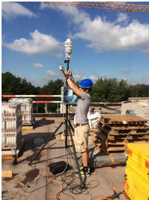
Figure 21 : Weather station on the roof
